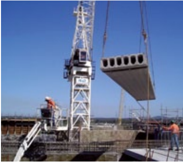
top: Hollowcore floor planks being fixed into position on a multi-storey deck
