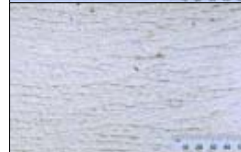
Figure 5: The exposed aggregate (top), broomed (middle) and wood floated (bottom) finishes, shown with a 50 mm scale.
