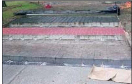
Figure 3: The concrete pavement was placed in two stages with dowel bars along all construction joints
