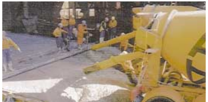
Figure 2: Pouring concrete on slag alley with the vibrating screed levelling the surface
