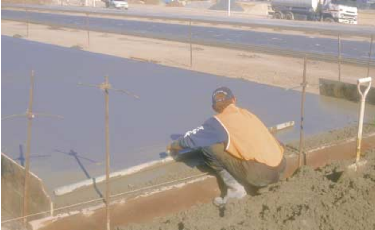
Figure 4: End board is installed, the gap filled and compacted and the surface screeded to the required level
