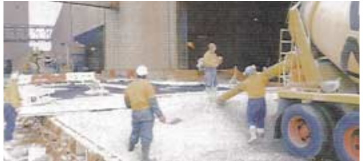
Figure 1: Placing concrete outside the steel melter with a fully laden steel kress in the background
