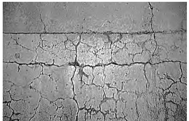
Figure 3.4 – Typical Map Cracking caused by Alkali-Aggregate Reactions
