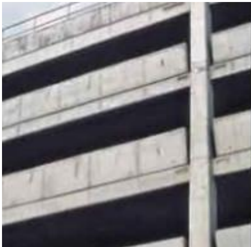
Figure 16.6 – Surface Marking due to Immersion Vibrator touching Formwork
