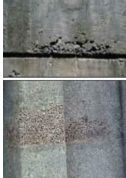
Figure 16.2 – Honeycombing due to Inadequate Compaction or Grout/mortar Leakage
