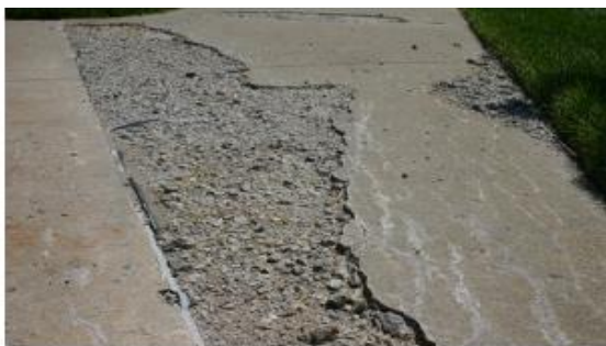
Figure 5.2 – Pavement Damage due to Freeze Thaw Cycles
