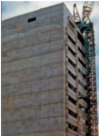
Figure 16.1 – Hydration Staining and Colour Variation from Concrete placed in Layers
